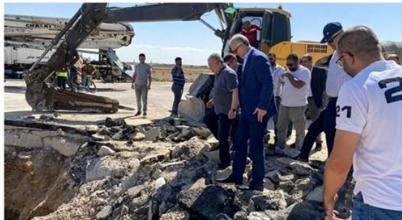
Syria's Prime Minister Muwazin Jzouzi inspects damage of the runway of Damascus International Airport on the outskirts of the Syrian capital on
